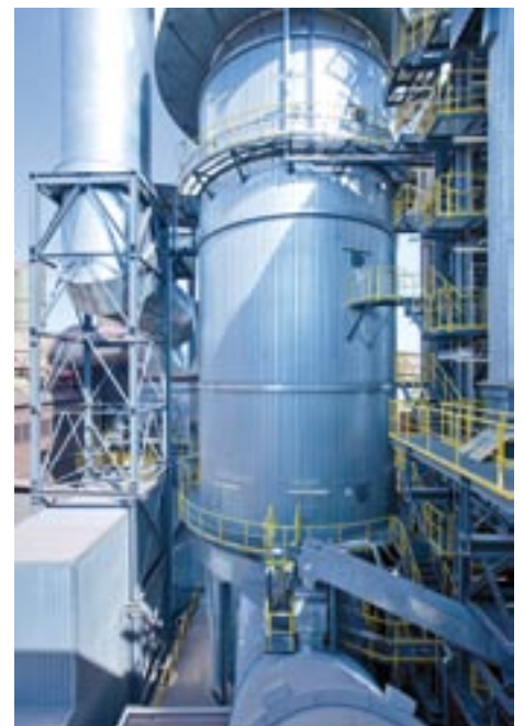
SIMETAL CIS MEROS gas conditioning tower
