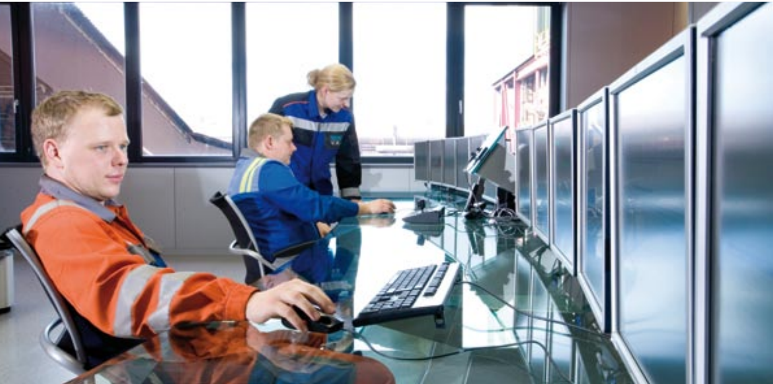
Sinter plant and SIMETAL CS MEROS ® control room
