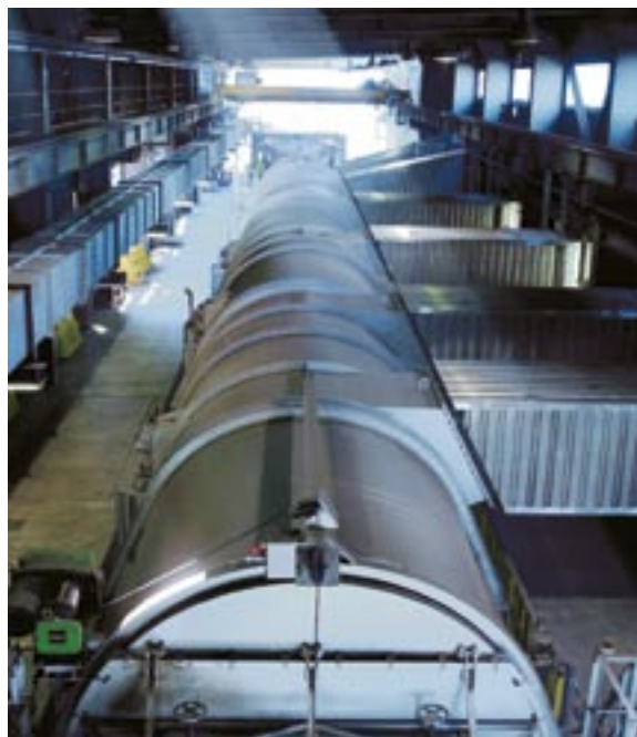
Sinter plant, voestalpine Stahl, Linz, Austria: Increase of sinter production and installation of the Selective waste gas recirculation system
