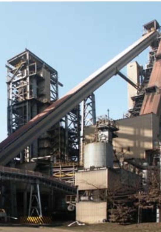
Hot DRI transport system
